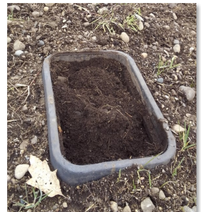
Hide-n-seek: Water meter box filled with dirt
