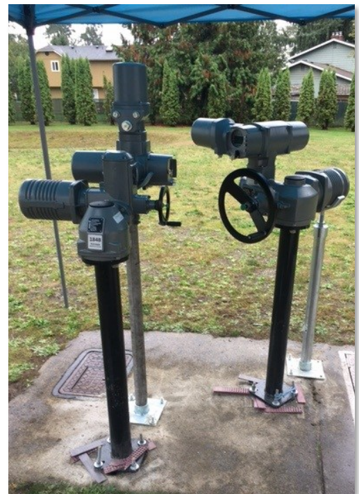
Pictured Below: Seismic valves at the Tanglewilde water system.
