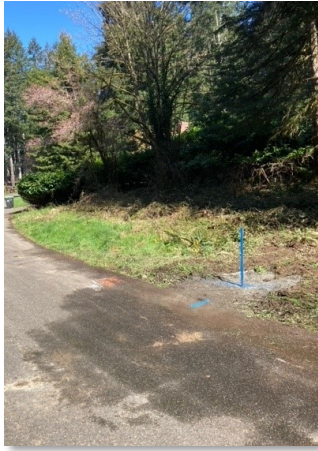
A wet spot on the road caused by a water main leak.
