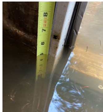
Five inches of flooding inside a pumphouse after a winter storm brought heavy rain.
