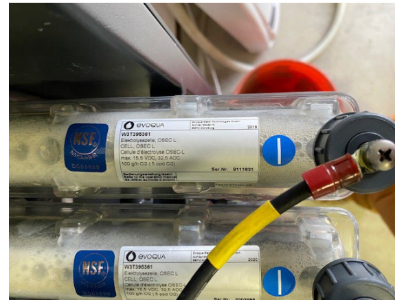
CL Generator Cells
