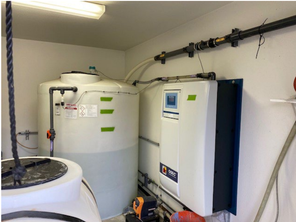
CL Generator and Storage Tank
